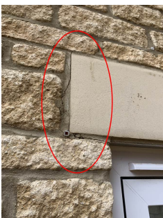
Repoint around lintels
