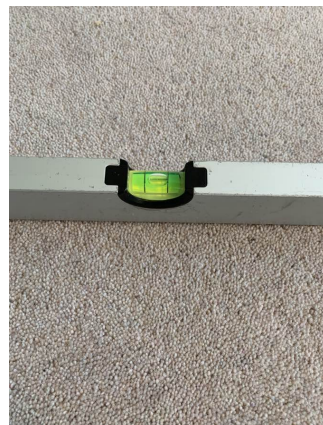
Floor not level btwn door & middle of room
