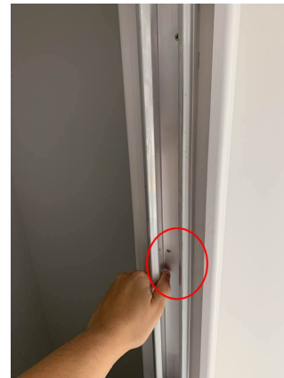
Screws missing from wardrobe door runner
