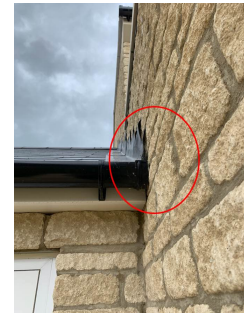
Flashing not flush
