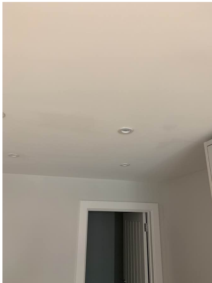
Paint flash on ceiling
