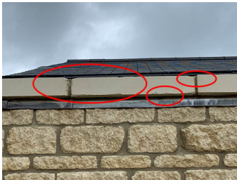
Coping chipped, sand coat
