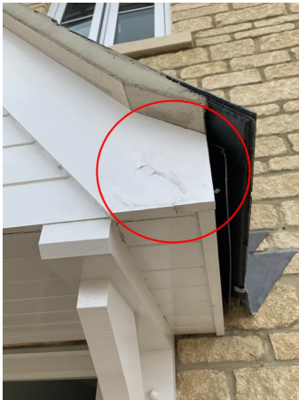
Paint damaged on canopy
