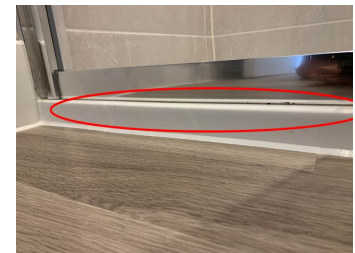
Sealant missing below shower frame
