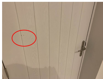
Damage on back door
