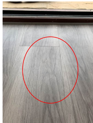
Floor scratched nr front door
