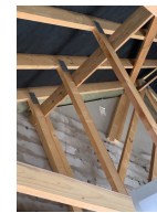
Firestop above wall loose, shouldn't be gaps
