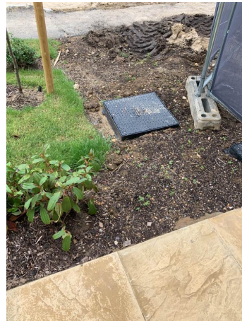
Front garden not finished
