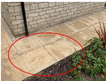
Slabs not level
