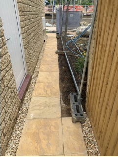
Fence not finished beside house
