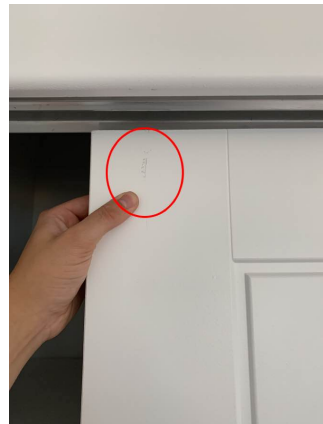
Blemish on wardrobe door
