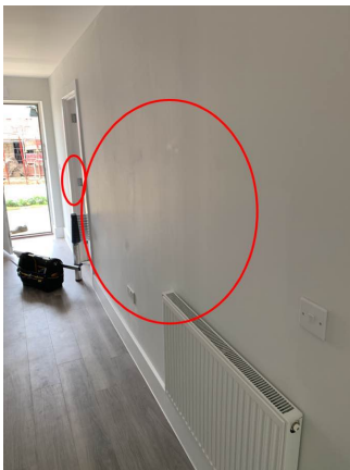
Paint flashing on wall, repaint
