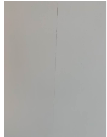
Board join crack on ceiling
