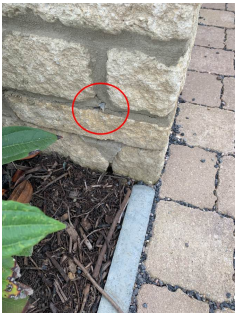
Weep vent damaged front corner
