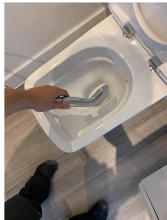
Shower head reaches toilet
