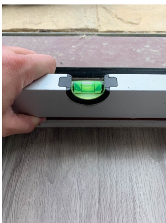
Front door threshold not level
