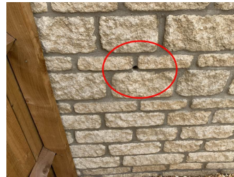
Hole on rear of garage
