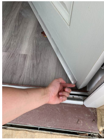
Weather bar end caps missing
