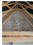
Mould on party wall
