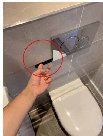
Poor tile alignment 2mm deviation
