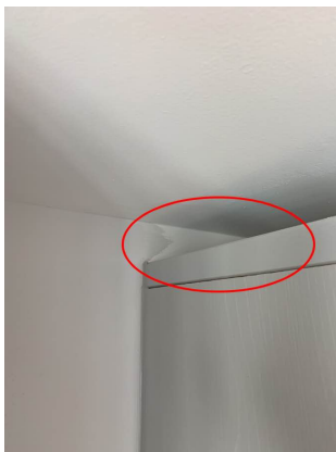
Paint missing above cupboards
