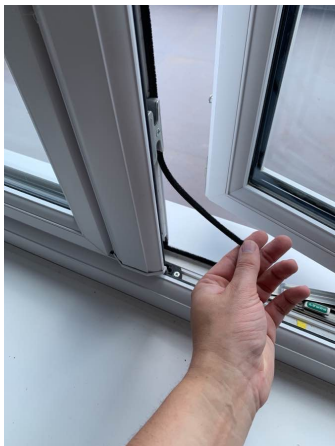
Seal loose on window
