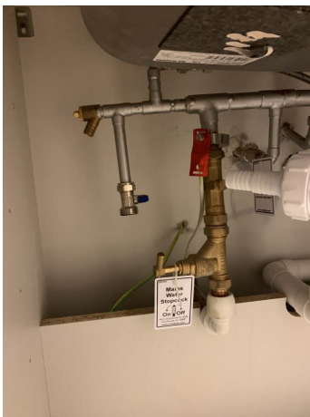
No double check valve
