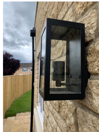
Some bulbs missing
