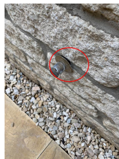
Sealant missing around pipe
