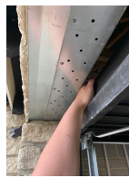
Pests could enter gap above door, cover
