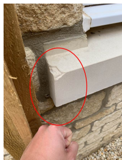
Cast stone damaged around fenestration
