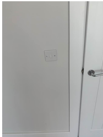
Switch not level
