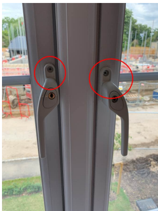
Pips missing from handles
