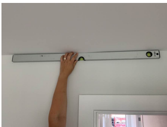
Ceiling not flat above door
