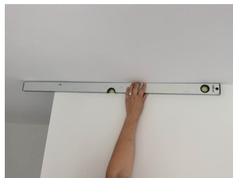
Ceiling not flat at inverted corner
