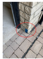
Membrane protrudes from brickwork
