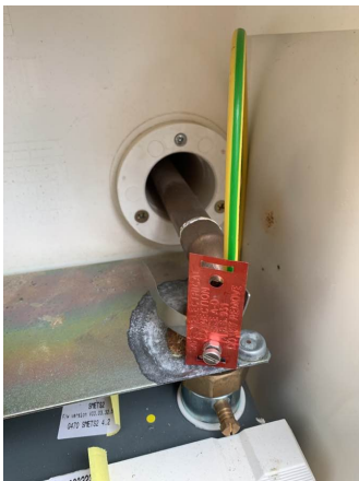
Intumescent putty missing from gas pipe
