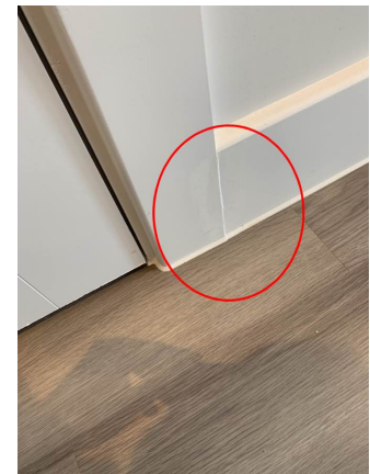
Wrong paint used for touch ups
