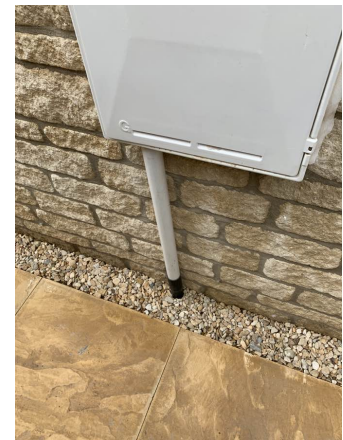
Gas pipe clip missing
