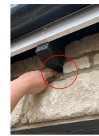
Mortar gaps around rafter tails
