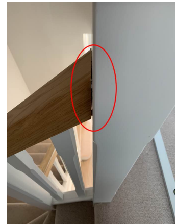
Make good handrail newel post joins
